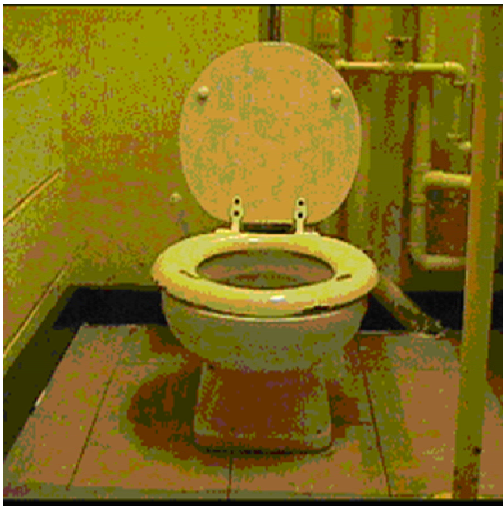
Figure 22.18. Baby Crane ® Toilet in Classroom's Restroom.
