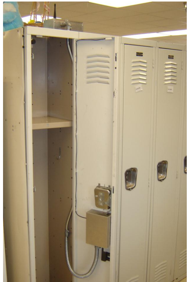
Fig. 8.23. Locker Unit and Power Supply.
